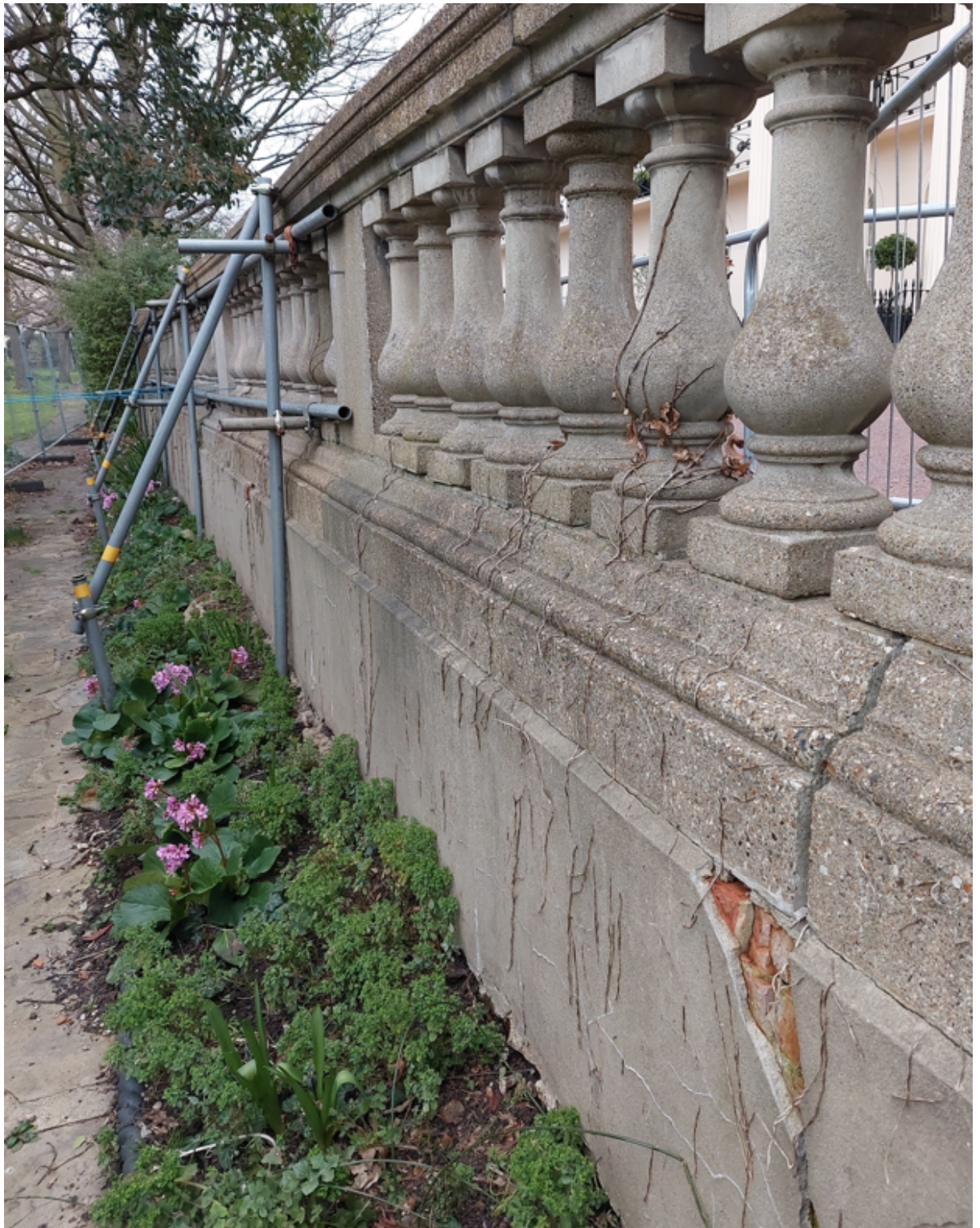
5. Existing wall with cracks being propped up by scaffolding and cordoned off by temporary gates
